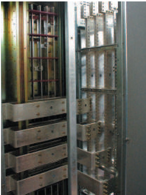
collegamento power center - motor control center connection between power center and motor control center
