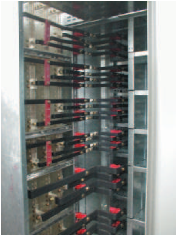
derivazioni tra calate e interruttori connections between secondary bus bars and circuit breakers
